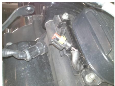
Fig 1.7 connect front O2 sensor harness and place plastic cover back in place.
