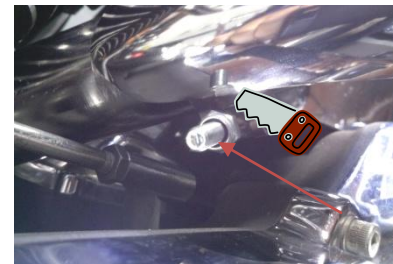
Fig 1.9 tighten T-bolt clamp and if you wish cut the end of the bolt threads flush with the nut
